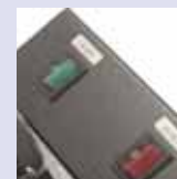
separate power and light switches
